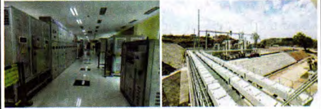
Fig 11. Controls and Switchyard
