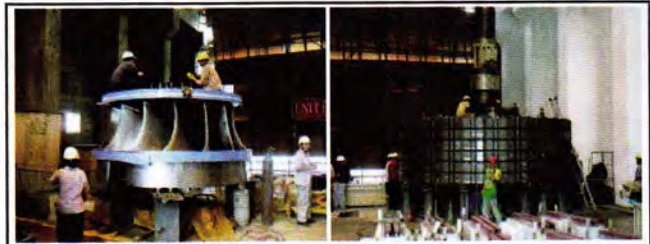
Fig 10. Turbine and Generator
